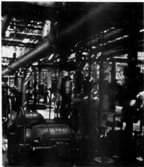
Corrosion and weathering doesn't harm G-E totally-enclosed explosion-proof motors. At Rock Island, the two G-E 40-hp motors of this type in foreground drive crude charge pumps, while the two G-E 15-hp vertical motors of the same type in background drive pumps charging partially refined oil directly to the cracking unit.
